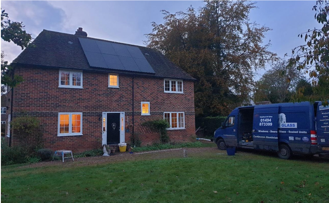
Above: Briar Cottage was the first cottage to receive a solar PV and battery installation, and it also benefitted from new UPVC windows to further enhance its energy efficiency
